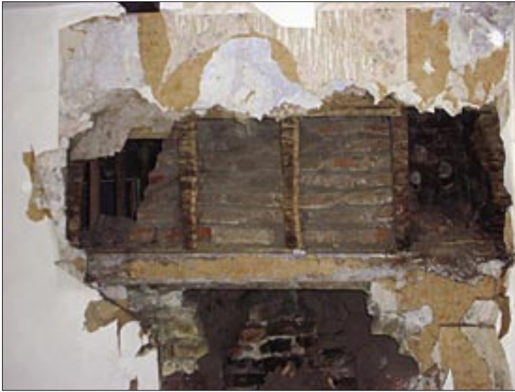
Figure 7 Chimney stack during demolition work; many items from the Sittingbourne Cache were found in the voids either side of the chimney stack.
